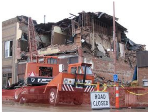
Demolition of several main street buildings and an old gas station at First and Walnut is now underway, with Brink Construction doing the work. Shown is the Rattray Building which once housed the news stand.
